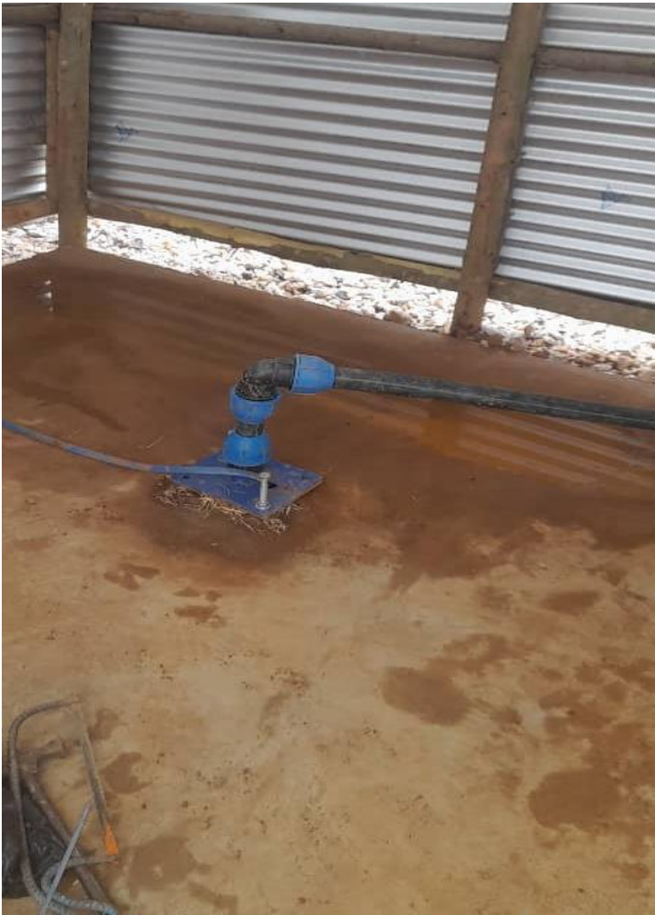
Submersible pump installed at H5 Resources Ltd, Ntungamo
