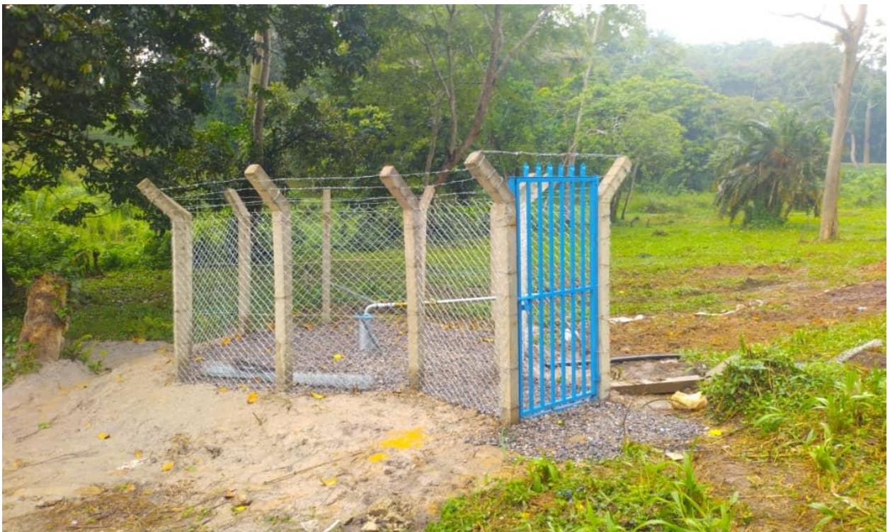
Pump fencing to prevent animals from accessing pump area.
