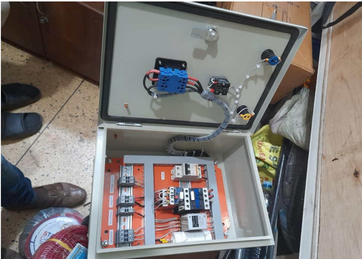
Customized pump control box built for submersible pump installed at H5 Resources Ltd, Ntungamo.
