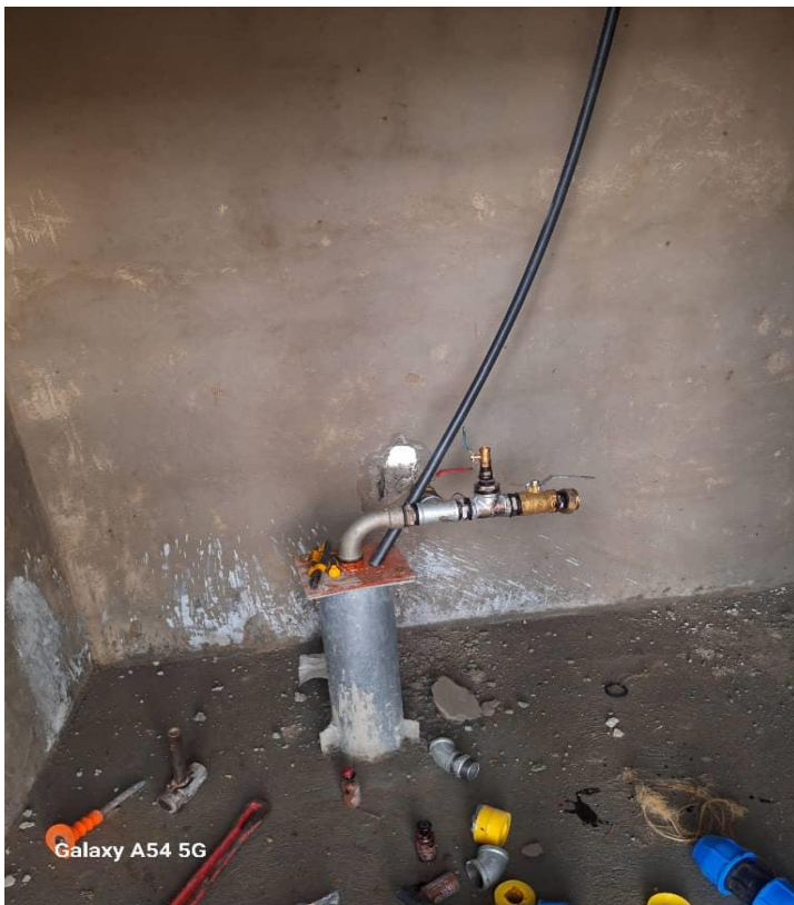
Pump installation in Ndejje University
